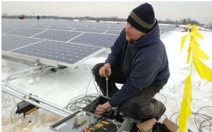
Journeyman Mike Carlon, with Swanson Electric company in Grant, works on wiring the combine box for the new solar panels on top of the Padnos Iron & Metal roof in Wyoming on Friday afternoon.
